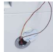
Cable port in the side wall
